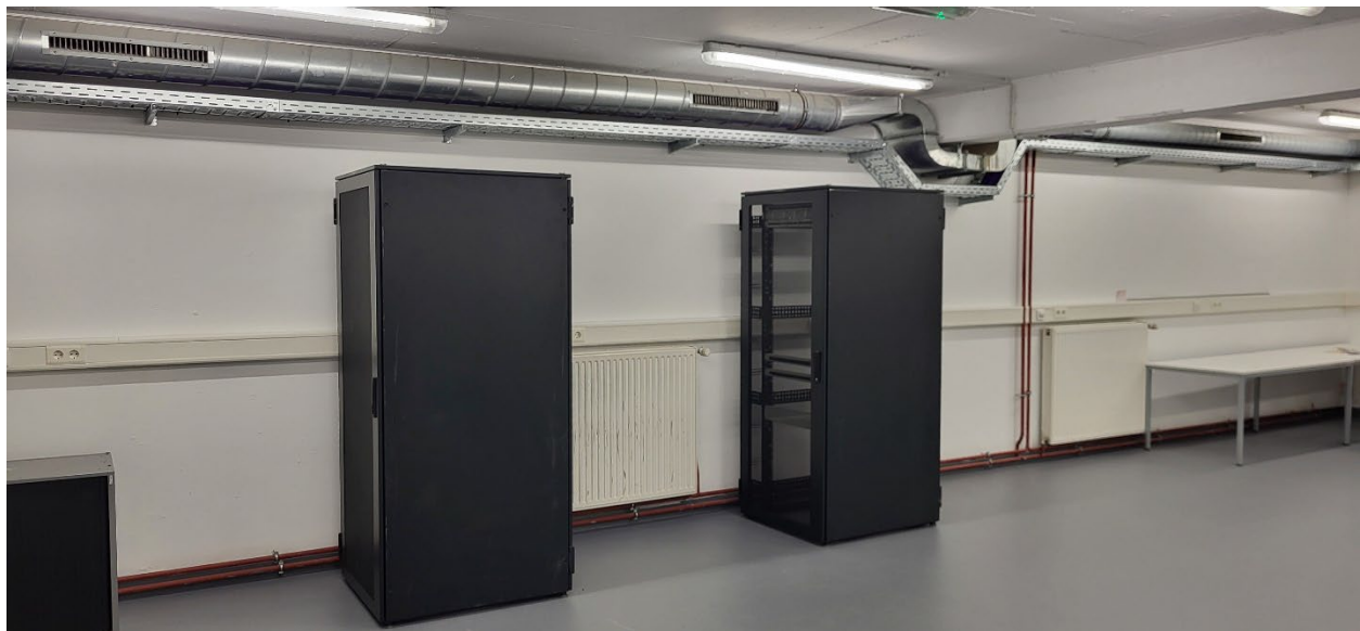
Figure 26. Rack placed in the Lab.
