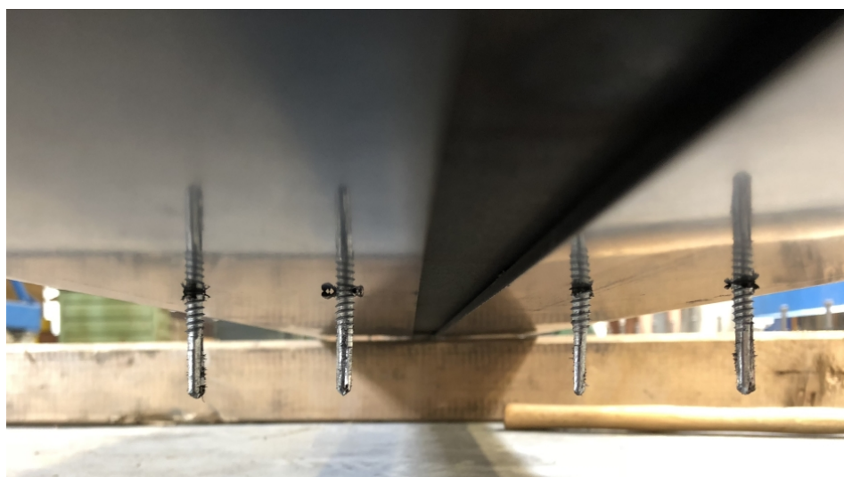
Figure 4.5 – The self-drilling screws in the “wrong” direction before being cut
