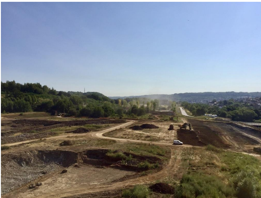
Picture 11: Decontamination and depollution work prior construction in Micheville, view from Belvedere, July 2018, Estelle Evrard
