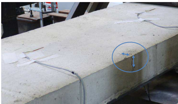
Fig. 16. Example of single cracks at the middle of the plate before loading (I-01-LS-0.75-TYPE A).
