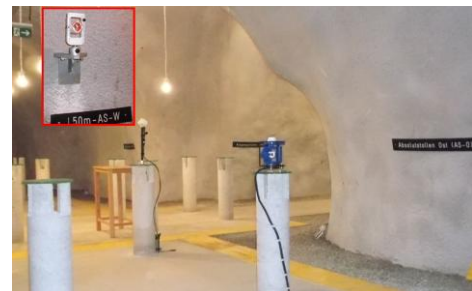
Figure 2: Installation location details. The insert shows a 50m distant corner cube, reflecting AUTODIF's laser beam. It is used as a directional reference.
